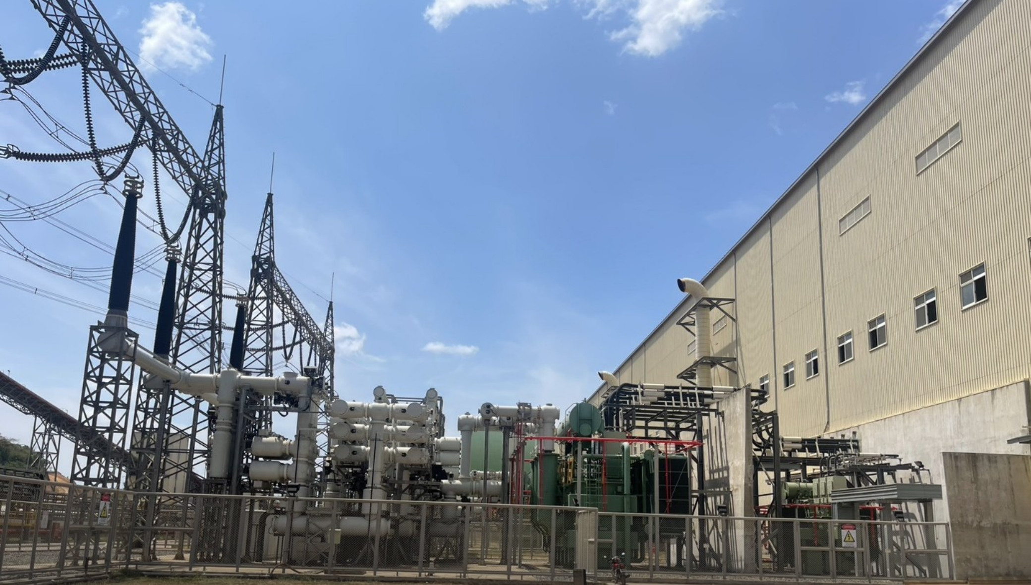
Mariveles 電廠變電站主變壓器設備，負責電力升降壓與電網銜接。 Main transformer facilities at the Mariveles Power Plant substation, enabling voltage transformation and grid interconnection.
